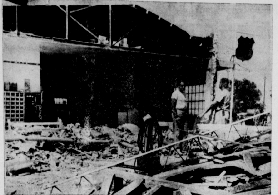
REMODELING AND MODERNIZING—Looking over the Springlake Motor Supply building is owner and manager Elroy Wislan as he talks with contractor Mal Burkett. Work started last Wednesday on tearing out the driveway. The remodeling job will include complete modernization of the front office, and to make a separate wash and grease room, also a double driveway in front, giving more room to service automobiles. Wislan said the job would be completed in about four or five week, but he plans to be open for business everyday throughout the remodeling process.
