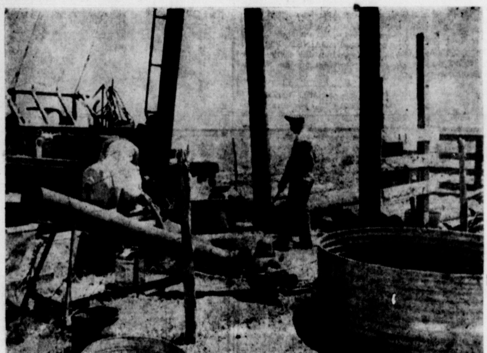
Above is O. D. Scheller and Cliff Holium employees of Brownd and White Equipment Co. as they work on a well using their newly purchased Service Truck.
