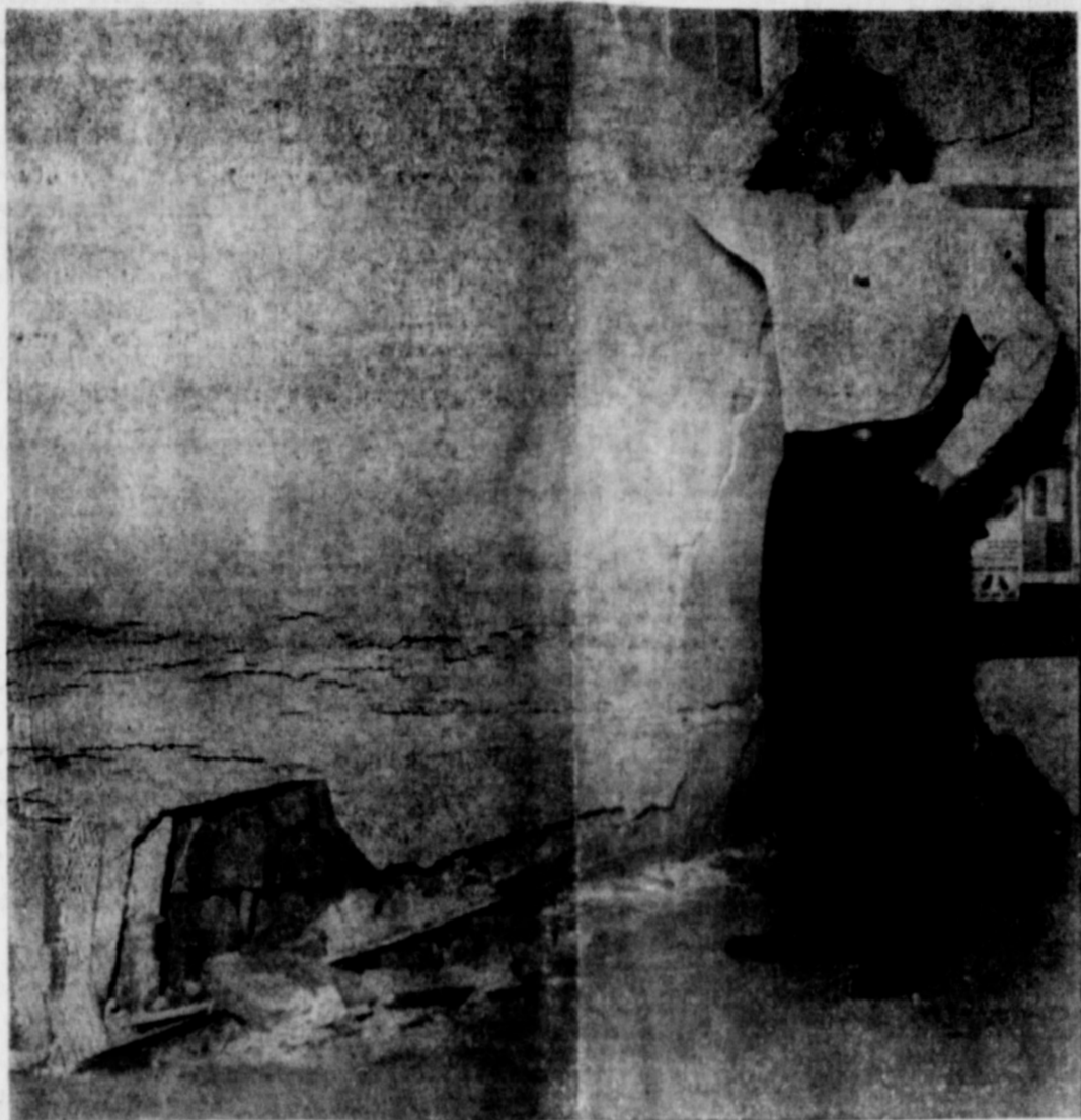
DRIVE IN POSTOFFICE — Postmaster Harold Miller is shown as he looks over the ruins of the modern new Post Office building Friday morning. Miller was busy with his duties when the crash took place, looking up he saw the walls were cracked and caved inward. Seems Earth
