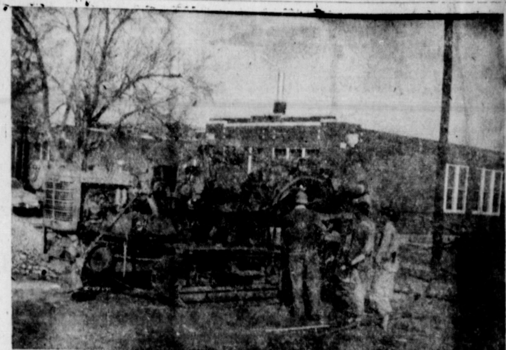
Workers were digging foundation trenches on the Springlake school grounds this week. The ditching machine is shown here as it started work on the new grade school building. It had already completed the digging for the addition to the high school. (News Photo)
