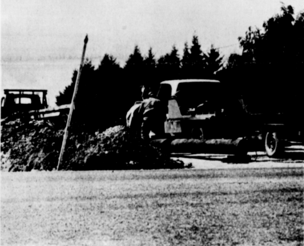
NEW WATER LINE-Goes under Highway 70 on the cemetery road, as part of the $85,000 city water sewer project.
