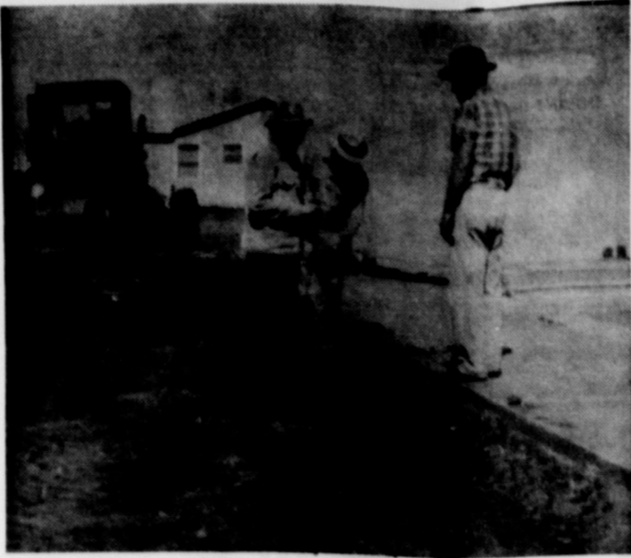
SWIMMING POOL TO HAVE BETTER FACILITIES — Shown above is Joe Davis and Joe Gilmore standing where new 20 ft. wide extension apron is under construction. W. F. "Dunk" Williamson is shown on original pool apron.
