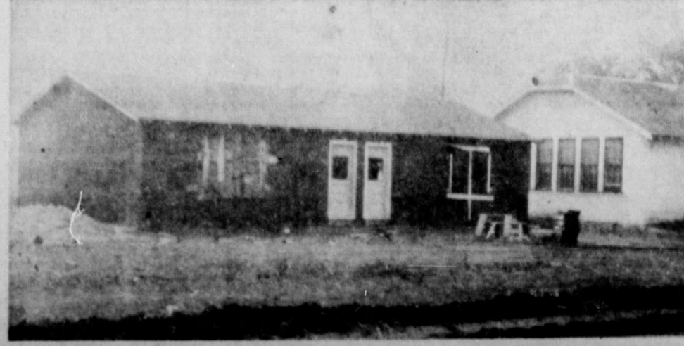
THIS IS THE NEW TEACHERAGE under construction at Springlake school across the road north of the main campus. Partitions will be left out for the time being so that it may be used as a classroom until new permanent classrooms are built. (News Staff Photo)
