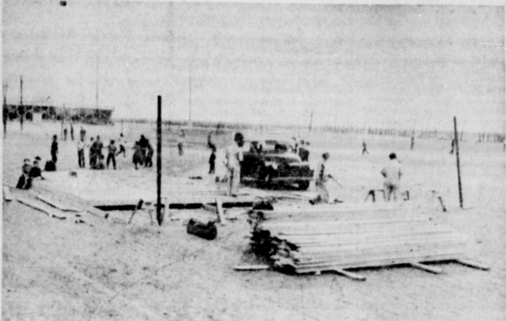
FOUR CARPENTERS employed by S. R. Duncan, Lubbock contractor, were at work at Springlake school building a tool house for the construction program. A week earlier employees of the contractor had surveyed and staked the foundation lines and they planned to start digging the foundations next Monday. Meanwhile everyone was expecting some sort of legal papers to be served on school officials to stop, temporarily at least, the work on the buildings. But so far as reporters could learn at press time Thursday, no such papers had been served. (News Photo)
