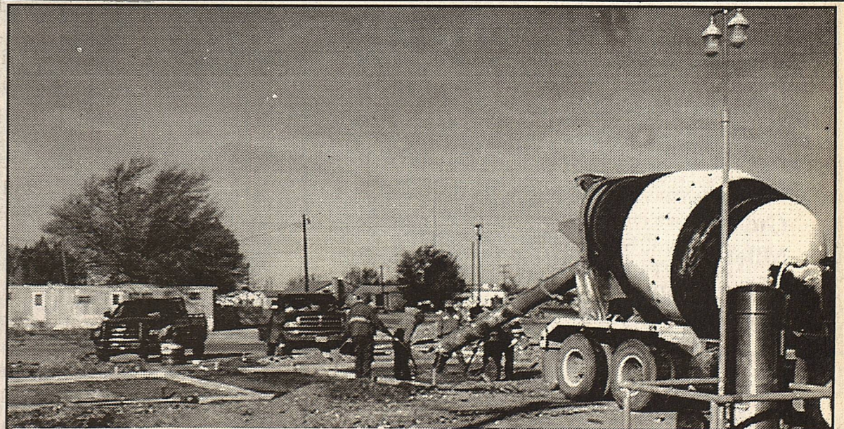
Workers were busy Saturday pouring cement for the floors of a new car-truck wash being constructed by Jack Spears. The site is on Cowboy Way, next door to Anne's Mini-Mart. Spears said the facility will have two large wash bays, one tall enough to accommodate full size trucks and tractors, and new equipment throughout.
