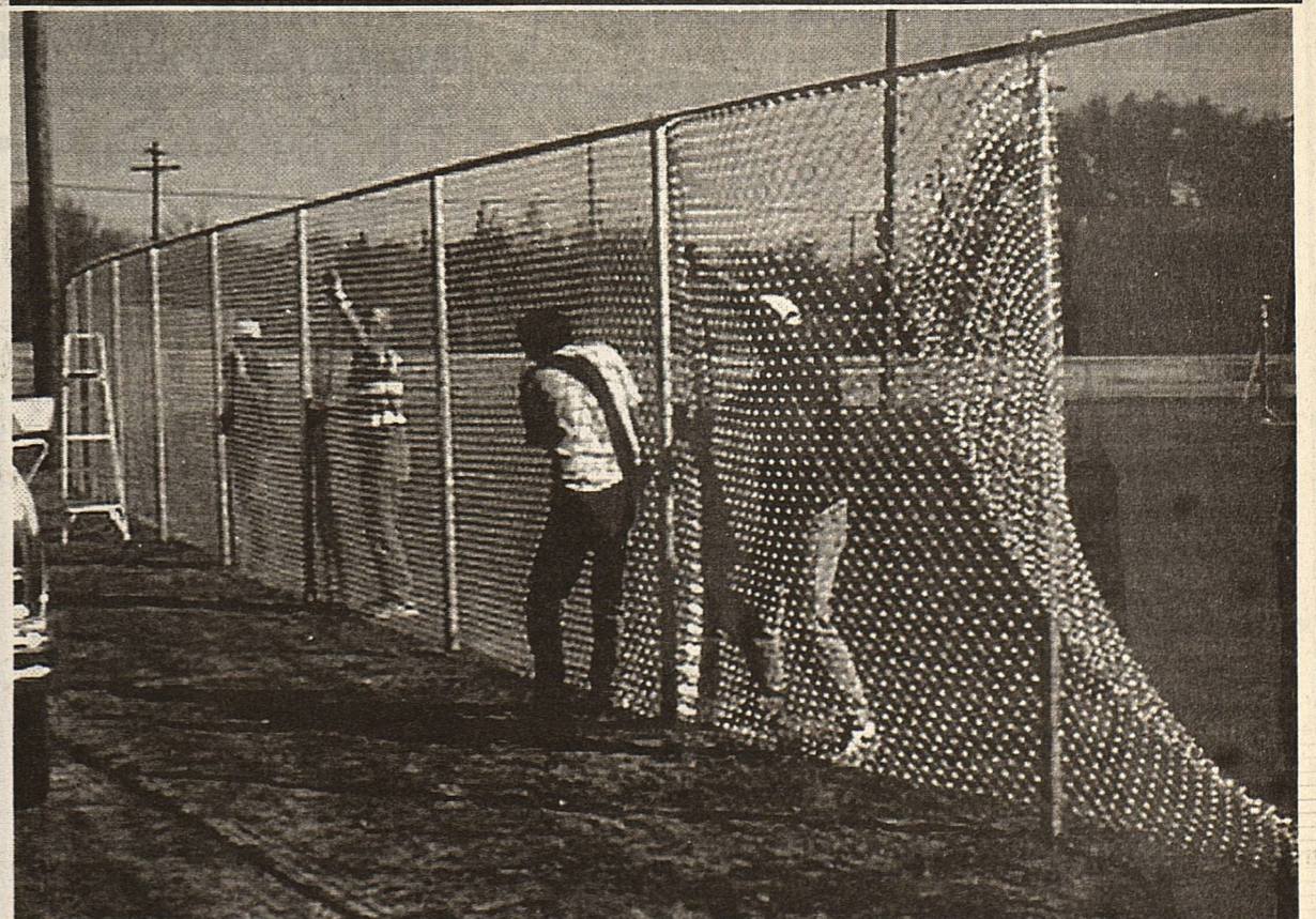
Construction crew shown installing new chain link fence around the new and very attractive high school baseball field.
