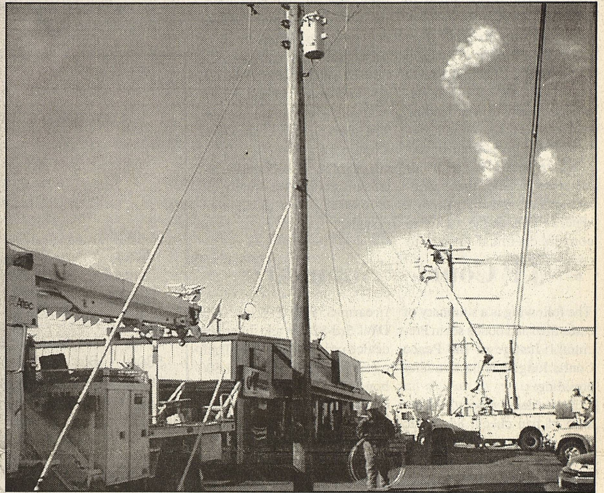
The electric pole in center of photo shown being removed last Thursday.
