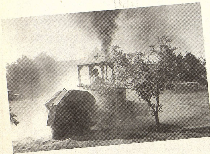
If you've been by the CSW campus recently, you can see that we're really shaking things up! In order to better serve our students and community and to raise the bar of quality even higher, CSW is undergoing major reconstruction which will increase total campus square footage by a whopping 68%.
