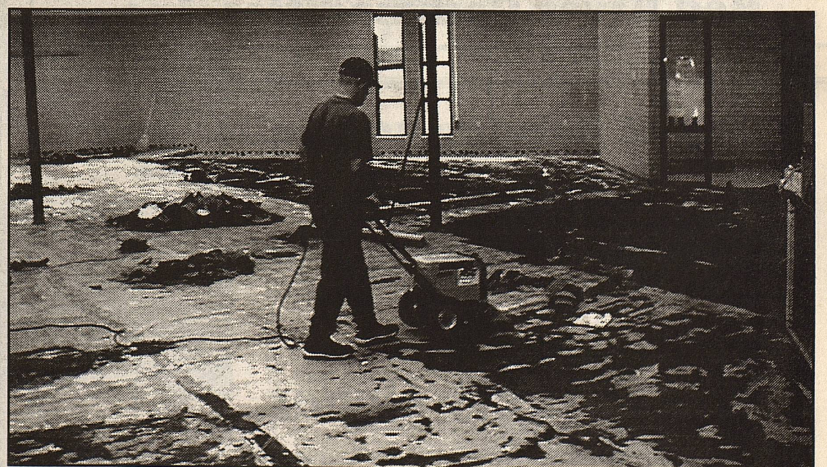
PISD employee Junior Lira busy removing adhesive under carpeting in the Resource Center
