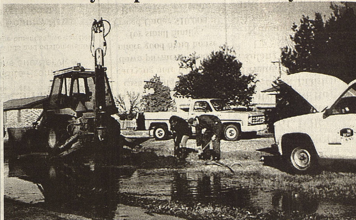
City employees Valentin Luna and Jerry Dominguez are shown last Sunday morning repairing a water leak in the city system in front of the Raymond and Marjorie Diaz residence. Before the cold and wet mainline repair job was complete, water had run from the site down Cowboy Way almost to Highway 214.
