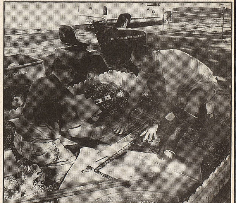
County employees Danny Steffens and Greg McCravery laying red, white and blue ceramic tile on a new concrete 'Texas at the courthouse square.'
