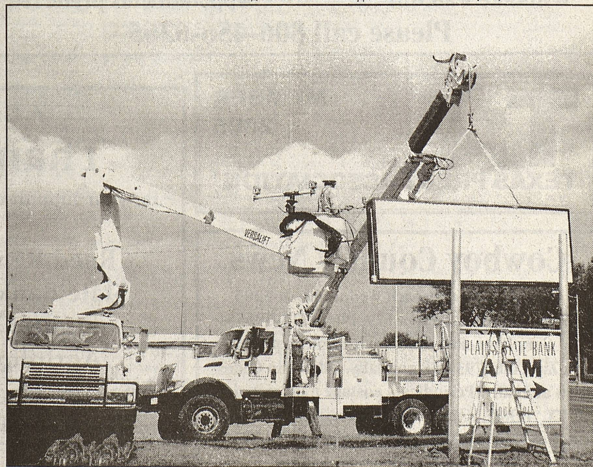
Lea County Electric Cooperative line crew members Manuel Estrada, foreground, and Gary Jones, background are shown on trucks used to remove the old marquee sign, to be replaced with a new electronic sign. Bill Rowe, who will install the new sign, anticipates finishing the job around July 1. Hundreds of commemorative bricks will be permanently installed around the new sign. The Cooperative will also help raise the new sign.
