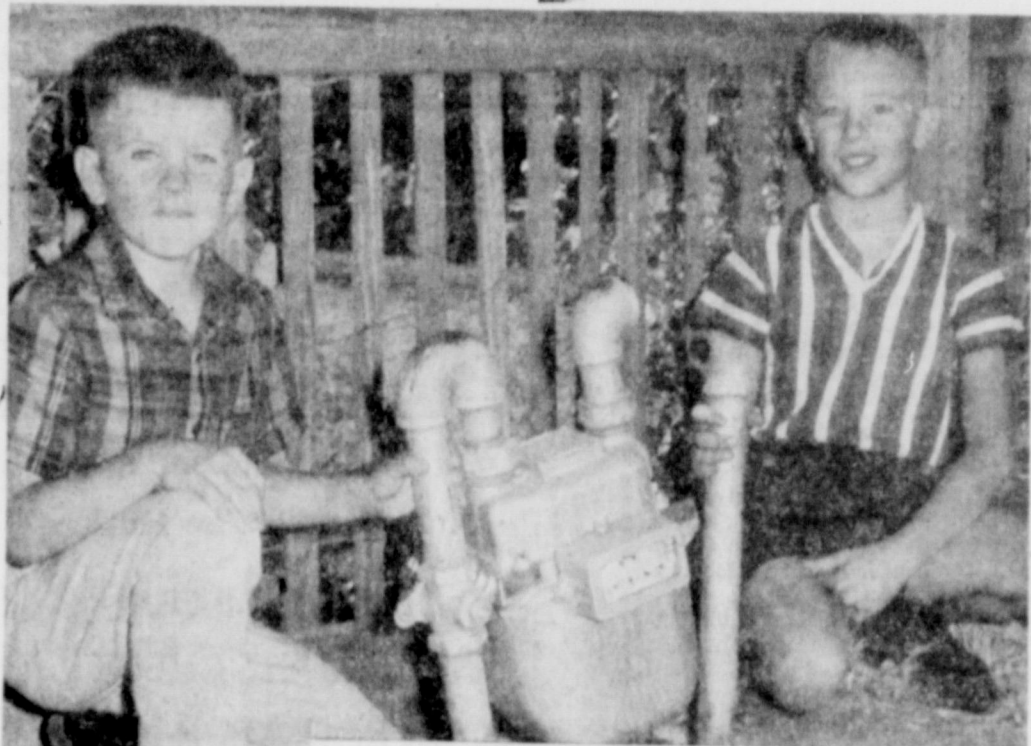
EXAMINE BROKEN LINE — Gordon and Matt Becker take a look at a broken gas meter which they discovered recently behind the Walter Kellum home at 240 N. 5th St. The boys, along with Jay Dunn, promptly reported the broken line to the gas company.
