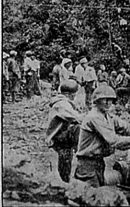
GOING UP —Korean laborers struggle up a mountainside with a length of cable that will soon be a part of an aerial tramway designed to ease the problem of transporting supplies to mountain troops. U. S. Army engineers (foreground) believe it will haul 400-pound loads on each 1200-foot trip in less than two minutes.
