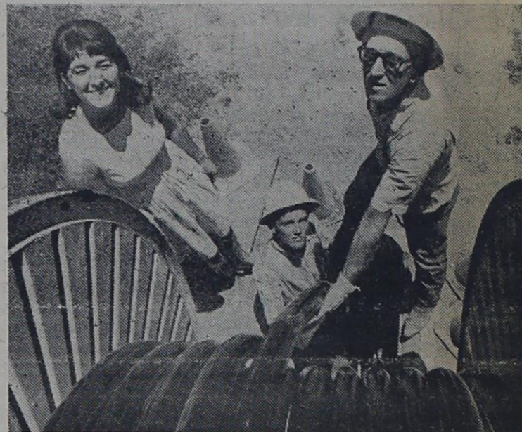
Pictured above is Miss Reda Pointer, Tech senior, as she watches a telephone cable being installed at Texas Tech. She is the daughter of Mr. and Mrs. J. C. Pointer.
