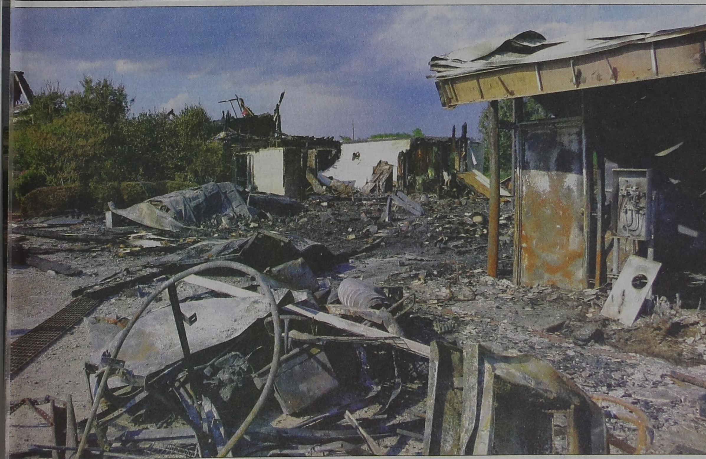
The fire-ravaged remains of this country house and business in Heath was a total loss due to a fire of unknown origin. The cause is under investigation. The shop to the far right and the garage was totally destroyed, as was the house, far left. Shown in the middle of the photo is a Lexus automobile underneath the melted garage doors. Photo by Millie Jean Coppedge/Rockwall County News
