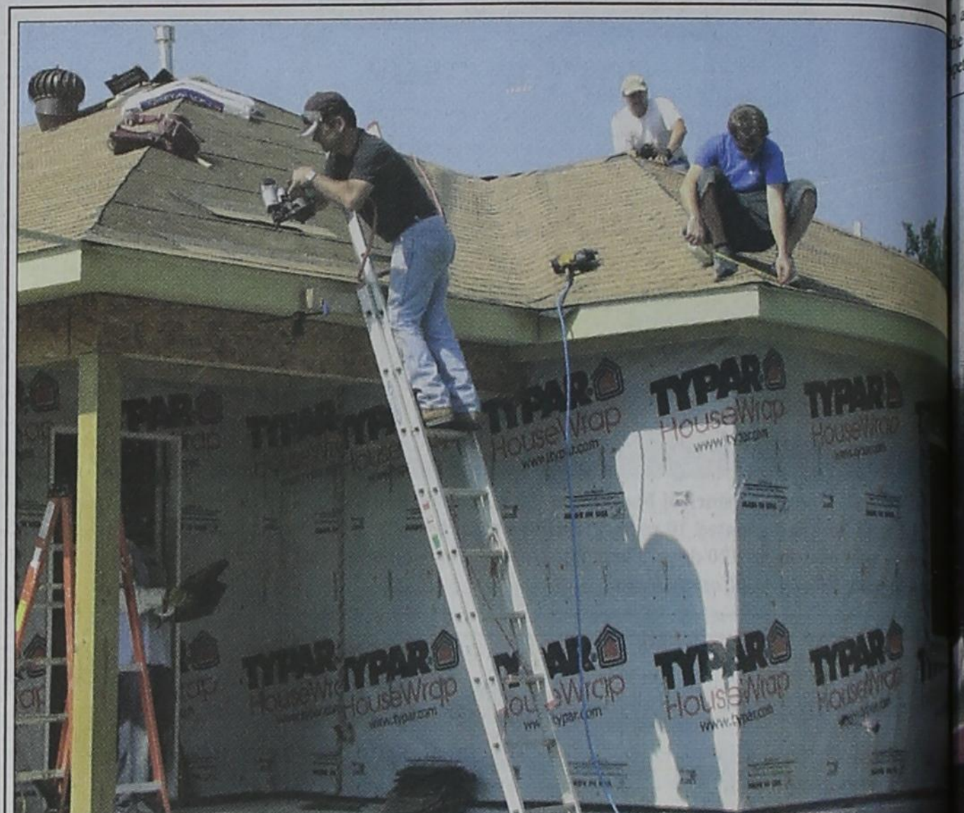
The roof of Rockwall's newest Habitat for Humanity home went on Saturday as crews laid shingles up top and continued inside the house framing walls. Construction on the house, located at 304 E. Ave., began in January. Helping with the roof were volunteers Steve Wood, on ladder, Craig Ledgerwood, center, and Jeremy Benz, blue shirt. To assist with this house or to make a donation, visit rockwallhabitat.org. Photo by Kathy Williams/Rockwall County News
