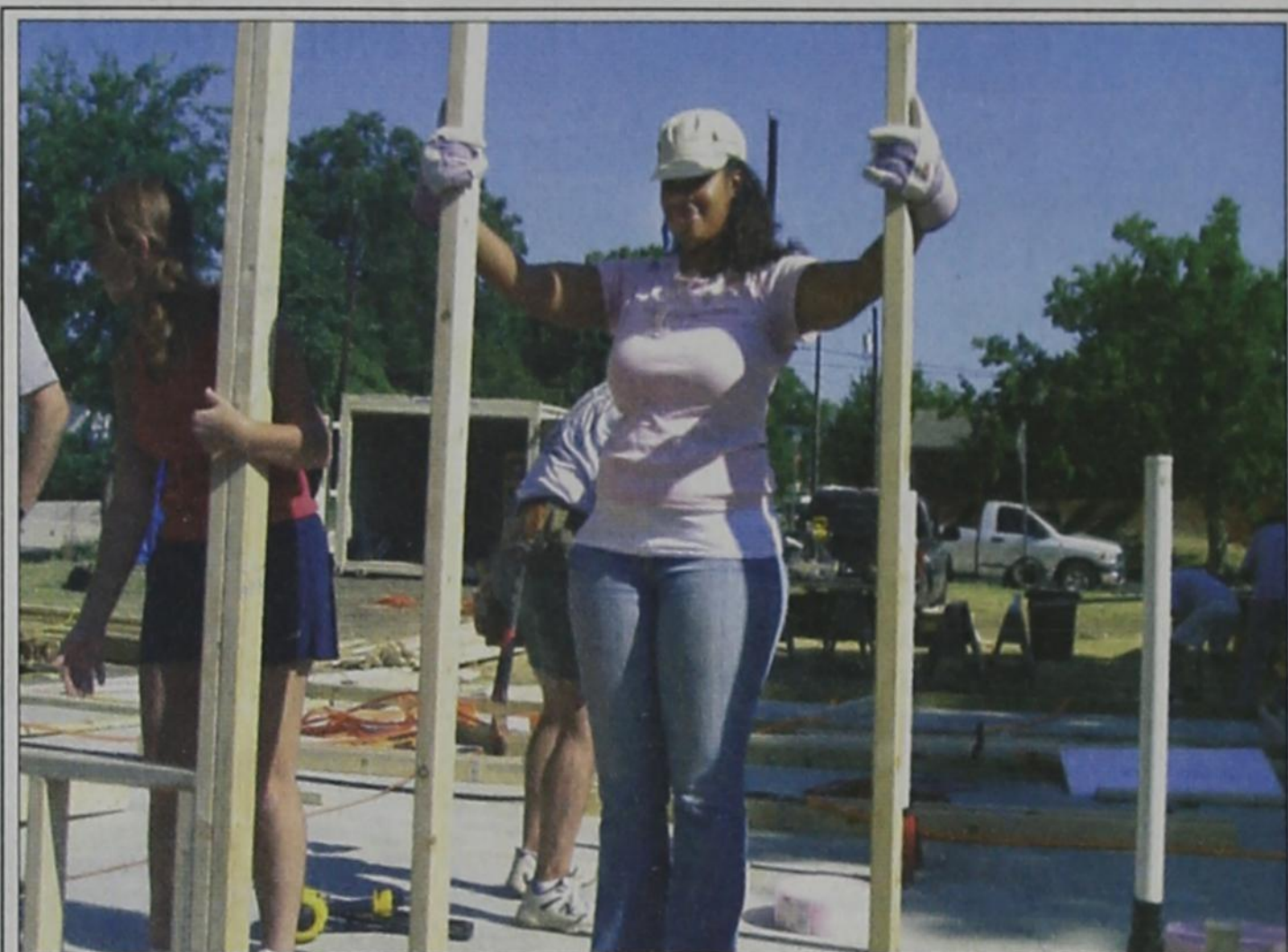
Homebuilder/owner Jessica Fisher helps to raise the first wall of her soon-to-be-completed home in Rockwall with help from volunteer Wendy Lawrence. Fisher and about 150 other Rockwall Area Habitat for Humanity volunteers have spent approximately 35 Saturdays constructing the dwelling, which Fisher is purchasing on a no-interest loan from RAHFH. Photo by Patricia Butts/Rockwall County News
