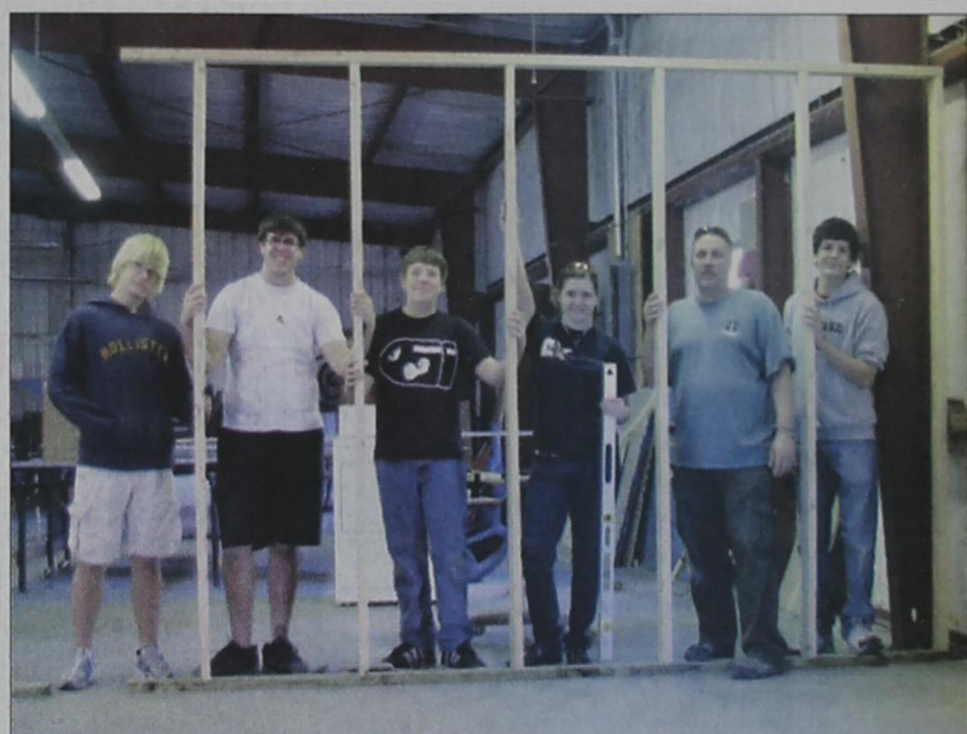
Kieffer Gilbert of Royse City (second from left), a Life Scout with Boy Scout Troop 690, completed a required project last weekend as part of the requirements to receive the rank of Eagle Scout. Gilbert and a group of volunteers walled in a 20x30 foot section of a warehouse at the First United Methodist Church in Royse City for the church's food bank. The church currently keeps its food offerings on open shelving but will be able to secure the food in the newly constructed room. All candidates for Eagle Scout are required to plan and carry out a leadership project that benefits their community, as well as fulfill several other requirements to receive Scouting's highest rank. Gilbert, who is also president of the Royse City High School National Honor Society and the Bulldog Guard, was joined at his project by his former Scoutmaster Scott Hammond, church trustee and project mentor Ben Fields, church youth minister Rick Ostrosky, church trustee Dean Gilkinson, as well as friends, family and fellow students from Royse City High School. Placing the first section of wall studs were (left to right) Gilbert's brother, Scott Mueller; Gilbert; brother Robert Mueller; friend and church member Heather Hebron; Ben Fields; friend and RCHS NHS member Ethan Downs. Photo by Kathy Williams/Rockwall County News
