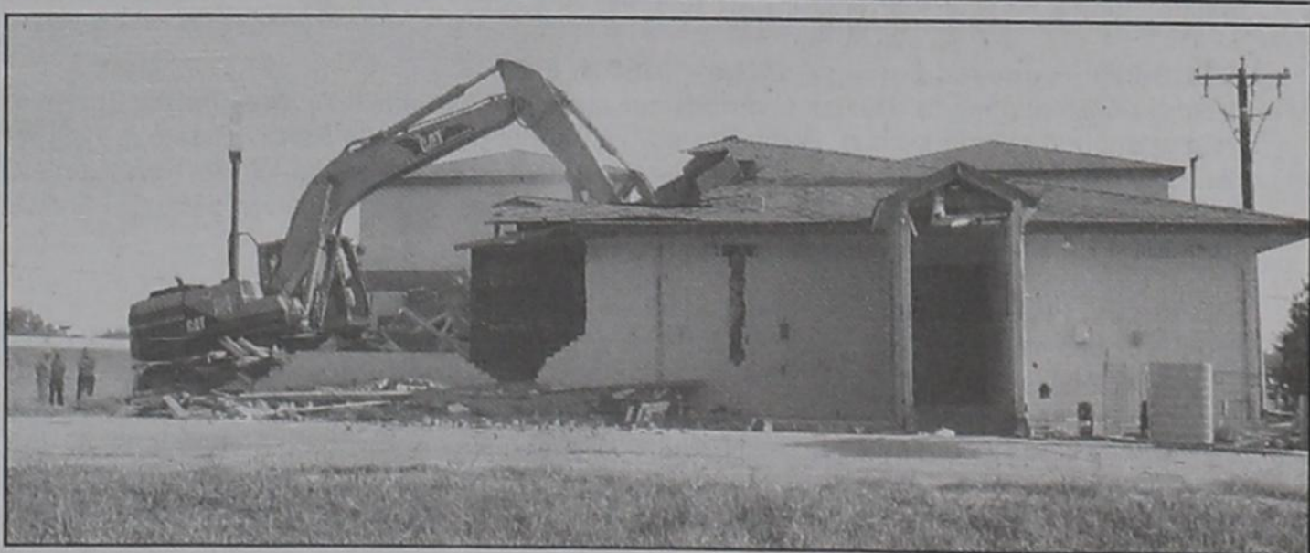
The former Royse City School Administration building, located 115 East I-30, was demolished Aug. 21 in preparation for the construction of a restaurant scheduled to open by the end of this year. Looking on as the building comes down are, from left, Larry Lott, executive director of the Royse City Community Development Corporation; Jim Hardin; and city manager Carl Alsbrook. Photo by Millie Jean Coppedge/Rockwall County News
