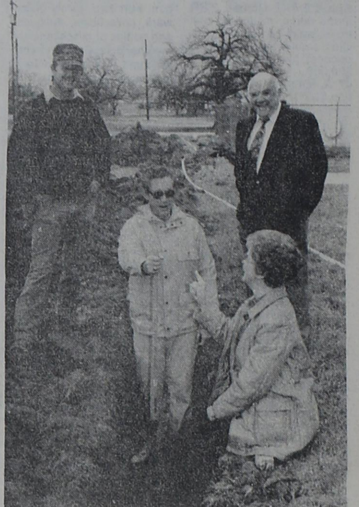
Rising Star City Council members, from left, James Cook, Edra Butler (seated) and Dr. Charles Barnes look on as Mayor Dr. Jerrell Bible uses a shovel in a utility ditch leading to the park pavilion, which is now under construction.
