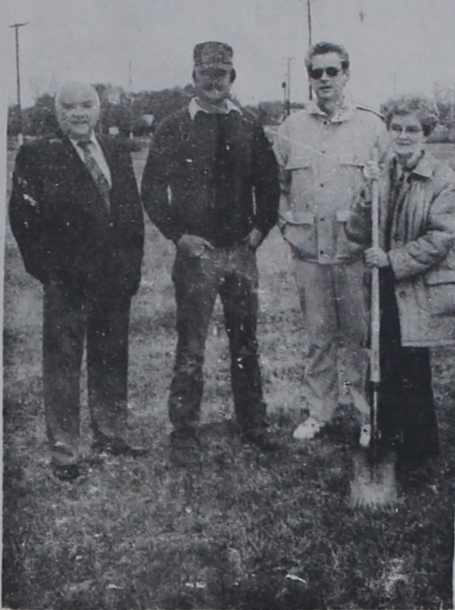
A groundbreaking ceremony was held recently to signify the start of the construction of a pavilion in Colquitt E. Williams Memorial Park. Present were Rising Star mayor and members of the City Council, from left, Dr. Charles Barnes, also chairman of the Park Committee; James Cook; Mayor Dr. Jerrell Bible; and Edra Butler, wielding the shovel.
