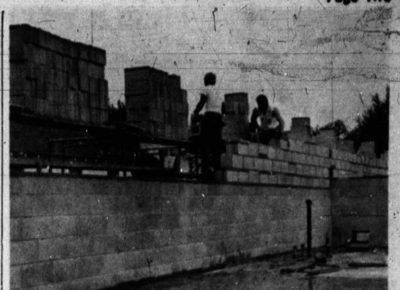
GOING UP — Walls on the addition to the Hereford Brand building at 130 W. 4th St. were nearing completion this week. The new addition will double existing floor space to the plant.
