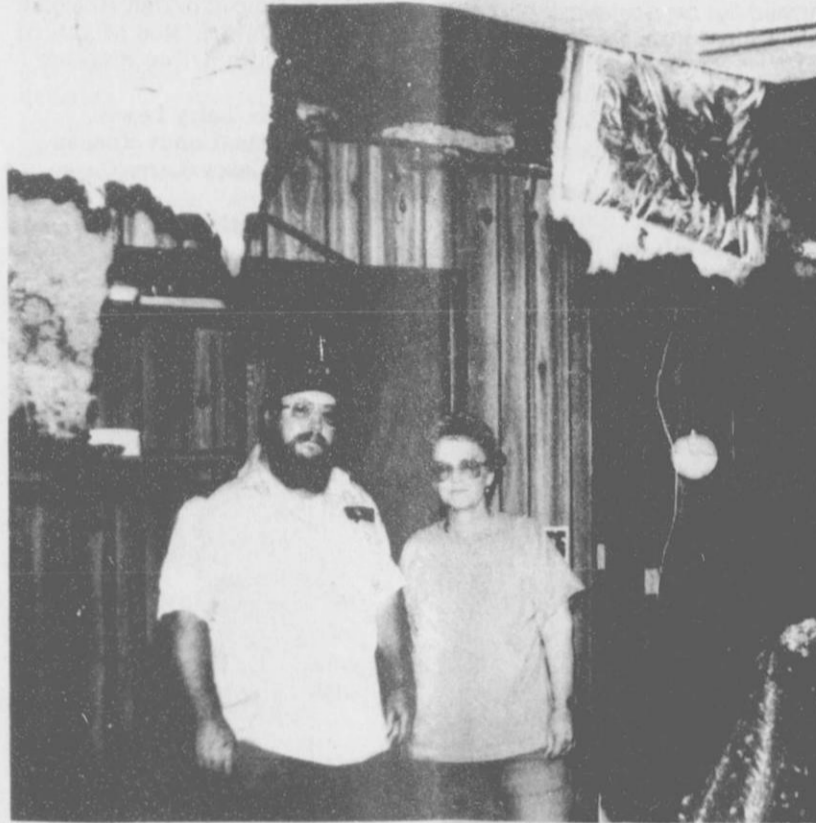
Fire Chief Sam Gruver, along with Peggy Dillow, inspects the damage done to Mrs. Dillow's bedroom ceiling by a fire Tuesday evening.
