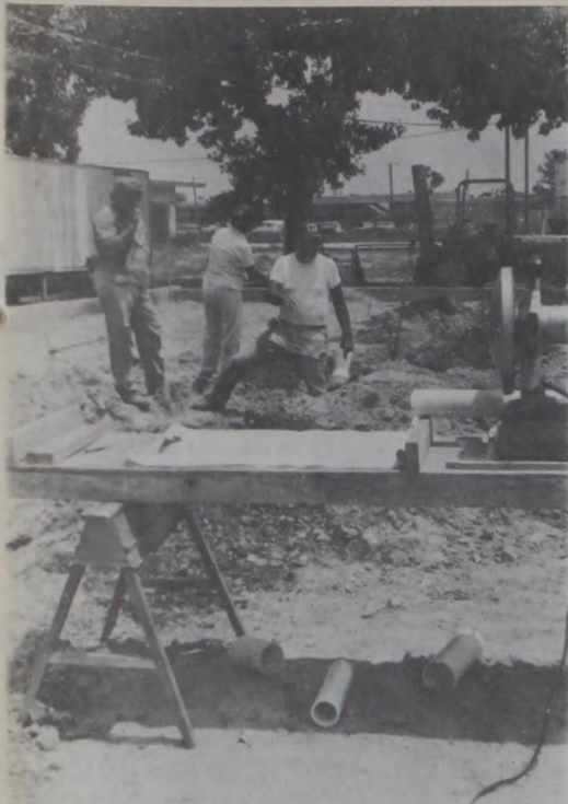
CONSTRUCTION at the new Center Restaurant is in the roughing-in stage. Plumber Earl Shasteen, his wife and helper, here, convert the plans on paper to the pipe works in the ground. Dave Fette Photo
