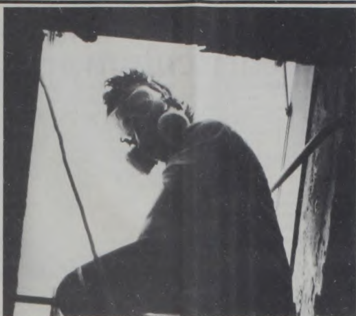
RANDY SCHOTT comes down through the trap door which lies at the base of the Sacred Heart Church steeple. He had just finished waterproofing the steeple with a toxic, naphtha-based compound which required the breathing mask and eye protector. Schott has worked with Leon Shabott for 10 years and is the only member of the crew that has not fallen at some time. He specializes in the steeple work. Dave Fette Photo
