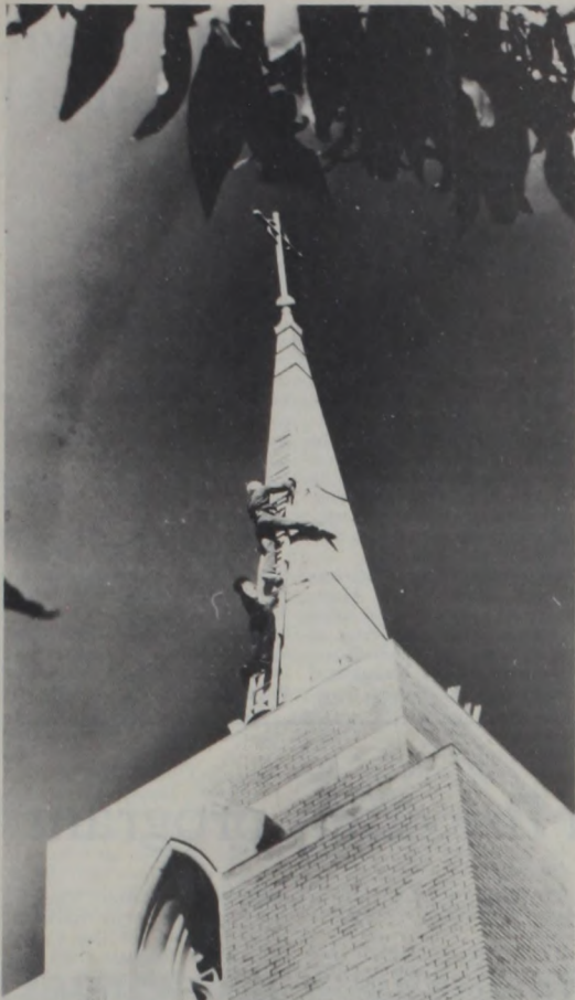
LEON SHABOTT, top, and Randy Schott, below, disassemble the special scaling ladder used while waterproofing the church steeple. Watch for more interesting photos next week. Janie Hartman Photo
