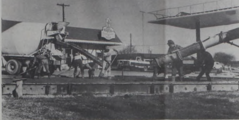
CONSTRUCTION IMPROVEMENTS nearly completed now at Bayer's Kolonialwaren include a new island, new pumps selling Exxon gas under a new canopy, and a new 30-ft. lighted Exxon gas price sign. Workmen are shown pouring the extension on the parking lot, which when completed will be approximately 200 ft. just east of the front entrance. The interior, explained Charles Bayer, will be enhanced with a seating area and booths near the front entrance for convenience of diners. Janie Hartman Photo
