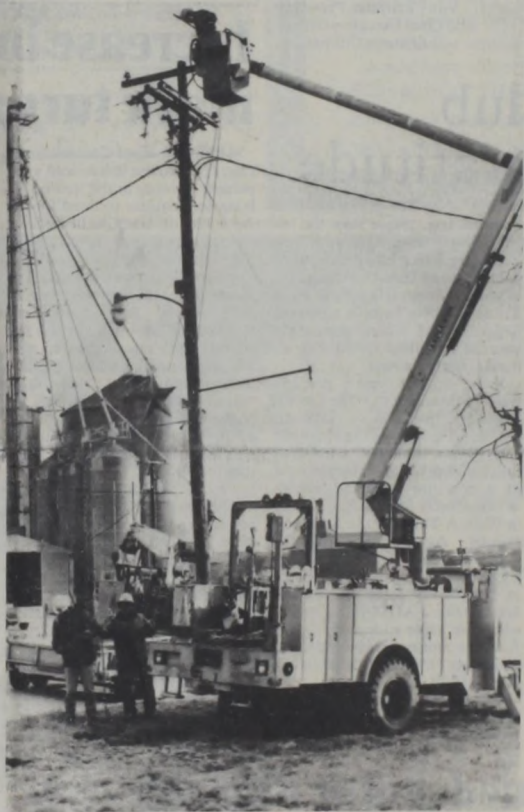
TEXAS POWER AND LIGHT CO. crewmen make repairs on the pole and equipment, quickly restoring current to the area. Tony's Seed and Feed Inc. elevators are in the background. Janie Hartman Photo
