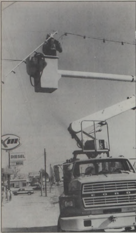
PETE PAYNE, member of the Texas Power and Light crew, connects the wires while installing the Christmas lights on Hwy. 82 and Main Street in Muenster last week. TP&L has been responsible for the lighted decorations for many years.
