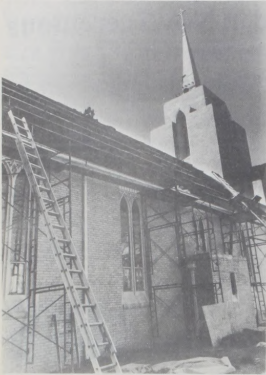
SCAFFOLDS on the north side of Sacred Heart Church through a wide angle lens. Workers on the top level of the steeple saw what you see below and at right.
