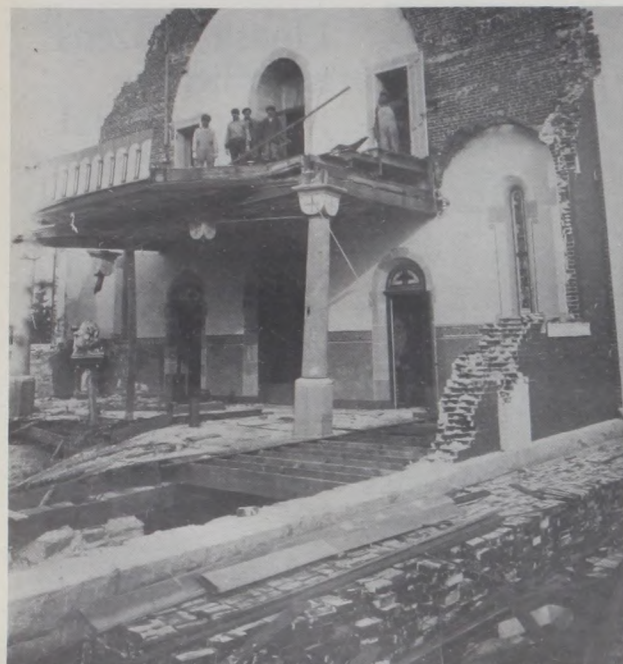
WORKERS BREAK to pose for a picture in the choir during cleanup of the church wreckage. Usable bricks were cleaned and stacked, in the foreground, to be reused. The tower was used in the present church, the front entrance was widened, two side doors and more reinforcement added for more strength.
