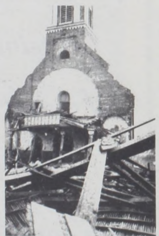
THE FRONT ENTRANCE AFTER THE STORM.
