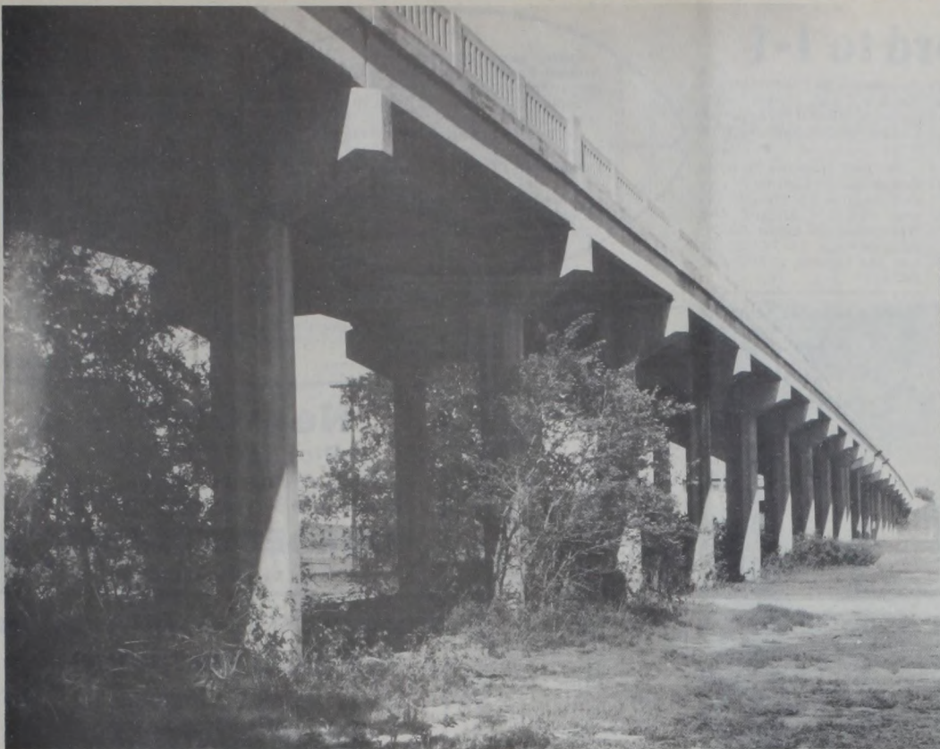
THE LAST SPAN of Muenster's new $90,000 overpass on Hwy. 82 was "completed this week," according to the Dec. 18, 1936 issue of The Muenster Enterprise . It was set to open to traffic on New Year's Day, 1937, but a spell of miserable weather delayed sufficient seasoning. This impressive picture is a copy of the original color photo made by the late
