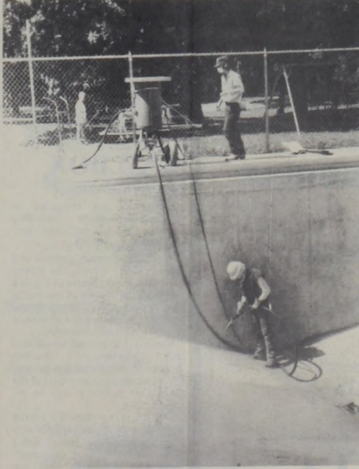
DOING AN EXTRA GOOD JOB of cleaning and painting the municipal swimming pool requires a few extra days to finish. Originally scheduled to open this weekend, the pool will have to wait till Thursday, May 29, for Splash Day. City Manager, Joe Fenton, made the announcement Tuesday.
