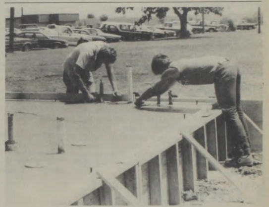
SAWING TIMBERS. Phil Walterscheid, above top, works at the sight of the new Young Children's Learning Center, scheduled for opening in the fall of '85. Wall sections started up early this week after concrete foundations and flooring were poured, smoothed and allowed to set. Above bottom, Charlie Knabe, left, and Neil Hesse, work through the heat of the afternoon sun.
