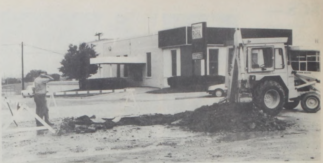
CHRIS YOSTEN, city water department employee, talks with Tom Swirczynski, back hoe operator, as they repair a water leak at the corner of Main and East First Streets on Friday. The 5:30 a.m. "leak" shot water approximately 30-feet into the air before city employees Garland Tate (not pictured) and Yosten were able to get the water supp-
