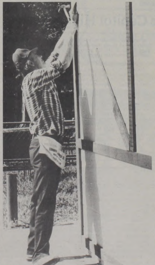
CARPENTER HAROLD KNABE secures trim on the side of the swimming pool building in the city park as part of an effort to clean up and dress up the town for Germanfest. The pool building, through the joint efforts of the park board, Chamber of Commerce and city, has been painted and trimmed to match the German motif of other park buildings. Photo by Janie Hartman
