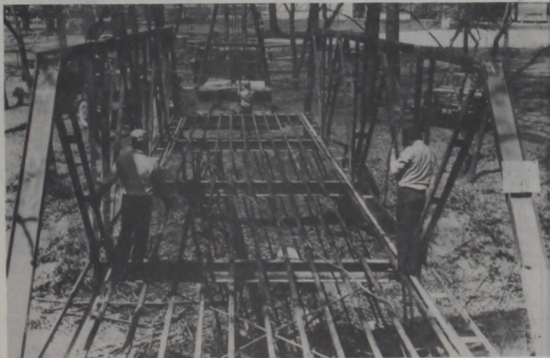
This new bridge across the Brushy Elm Creek in the city park will add a whole new dimension to a leisurely stroll during quiet times and greatly increased foot traffic capacity for the Germanfest.
