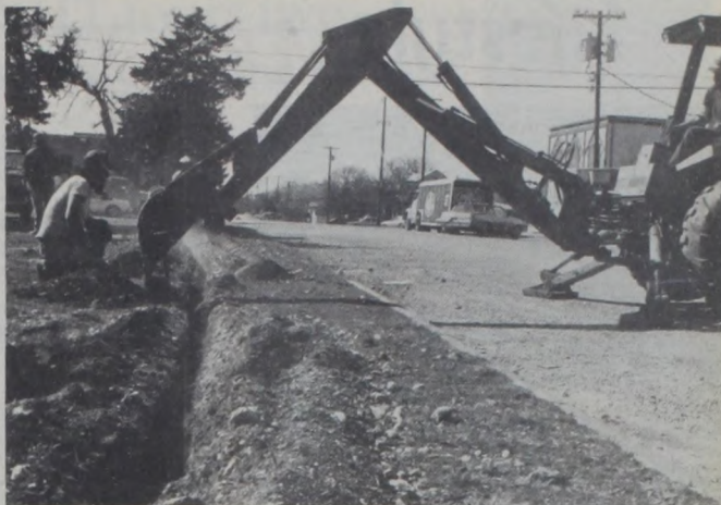
Construction workers on contract to the telephone company here work near Fischer's Market Tuesday, preparing the groundwork for installation of underground telephone cable. Workers said their contract calls for laying some 40 miles of phone cable in the Muenster area this spring.
