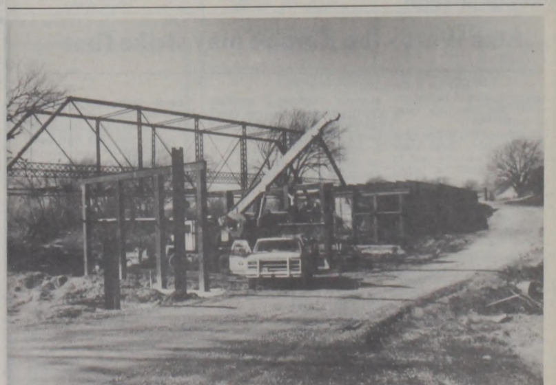
Construction continues on a modern new bridge south of Myra. The bridge spans 144 ft. In this photo by Janie Hartman, employees of Precinct 3
