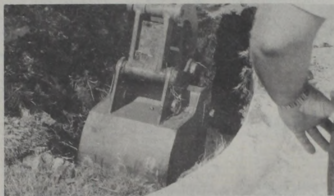
While Bell System employees are on strike in many areas, the construction continues for independent workers. In the above photo, Lehnis Perkins operates a backhoe (shown below) at the Muenster Telephone Company's current expansion project as Larry Eldridge looks on.
