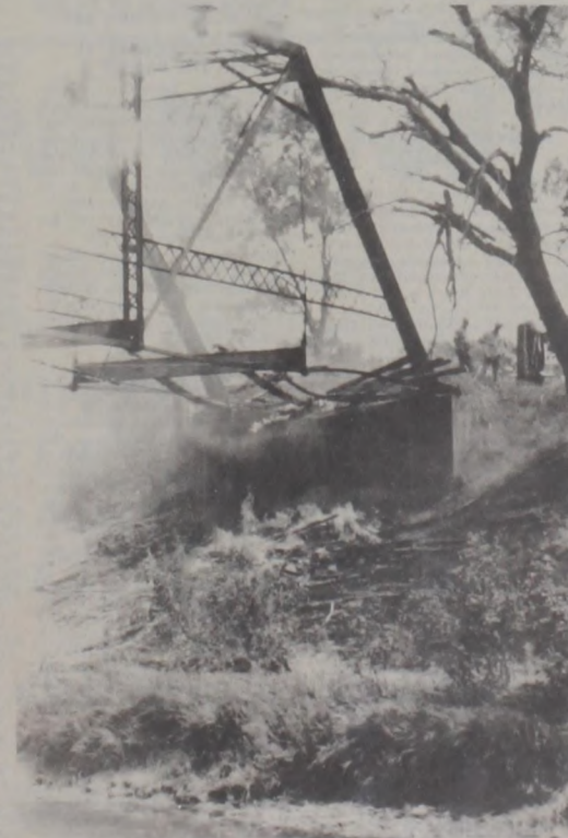
A SMALL PART of the remains at the bridge fire last week Friday at Elm Creek southeast of Myra. Damage consisted of warped steel and complete loss of flooring.
