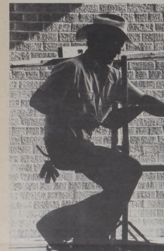
A BRICKLAYER AT ERA is silhouetted as he works to completed a doorway on the school's new addition before the start of classes. Photo by Bob Buckel
