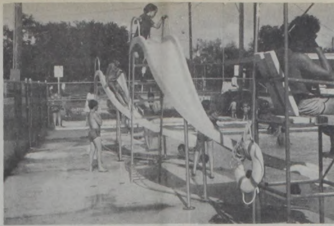
Staff Photo Kids at the swimming pool are enjoying these new water slides purchased by the Muenster Chamber of Commerce out of Germanfest revenue. Sam Endres and Roger Taylor installed them.
