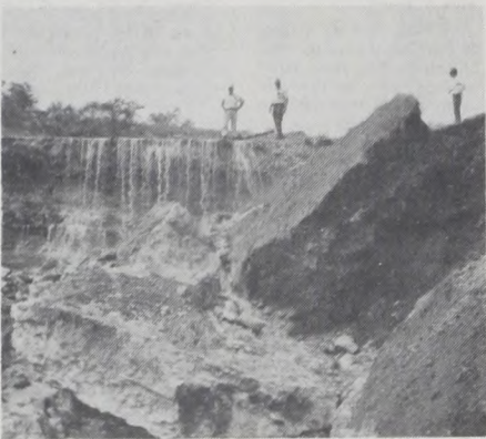
SCS Photo This washed out portion on the spillway of the Campbell Ranch Lake is one of many of destruction following last year's big flood. Seventeen flood control dams of the Muenster area were damaged.
