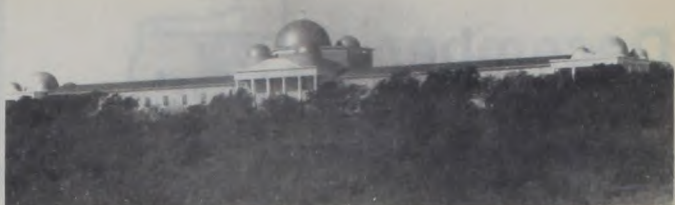
The exterior of the TM center is close to completion with the staff members there doing most of the work finishing the inside construction of the multi-million dollar educational facility.
