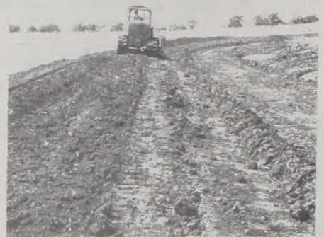
Conservation contractor using bulldozer to build broad based, easy to farm, channel type parallel terrace. Terrace dimensions are designed to fit the equipment used by the farmer.
