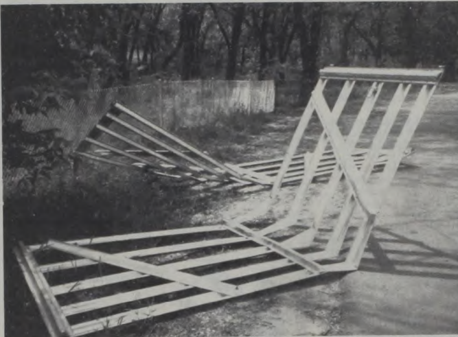
Vandals did this to a brand new metal gate just installed at the city park for Germanfest. It is only one many recent cases of property destruction. Staff Photo
