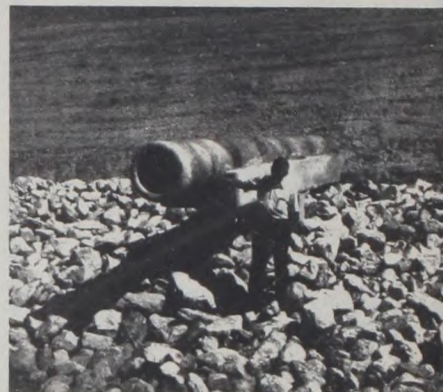
Pictured are the newly finished dam and principal spillway on Site 13C, Big Sandy Creek Watershed and the outlet pipe for the principal spillway on Site 13A, Big Sandy Creek near Sunset in Montague County. Two additional sites are under construction in Wise County near Rhome.
