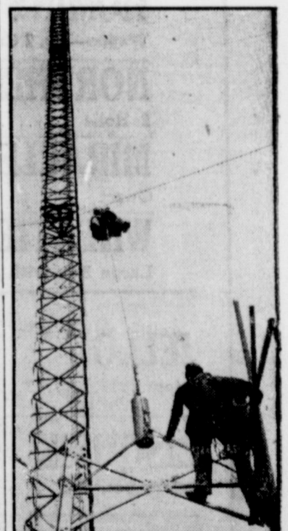
HIGH, CLEAR VOICE—Preparing for any possible complete severance of communications between Western Germany and West Berlin, workmen ascend a 450-foot very-high-frequency tower at Heckschorn, in Western Germany, to prepare it for transmission. Heckschorn station can route messages throughout Western Germany.
